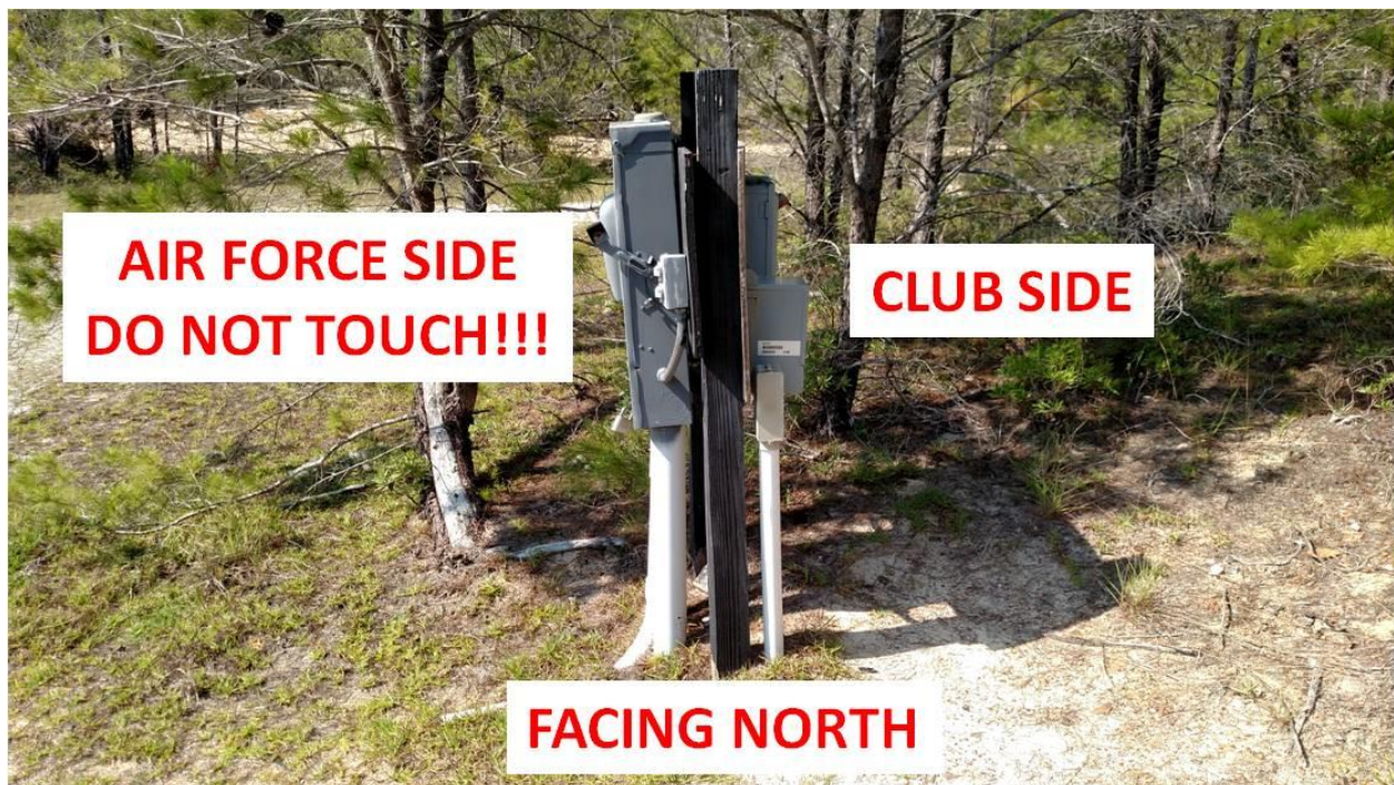
Figure 1 Electrical Junction General View
