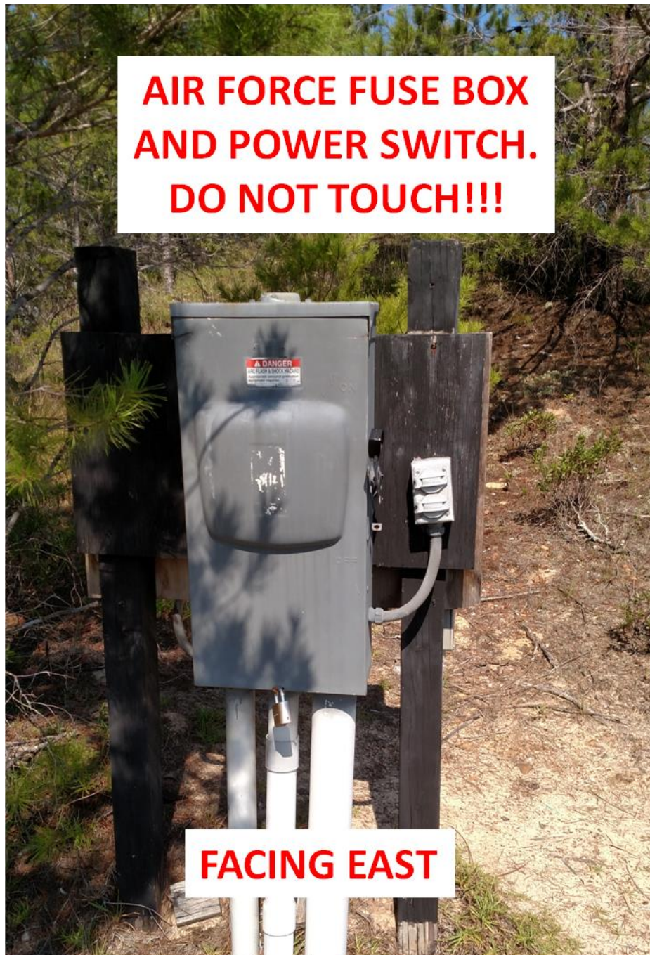
Figure 2 The Air Force side of the power junction.
