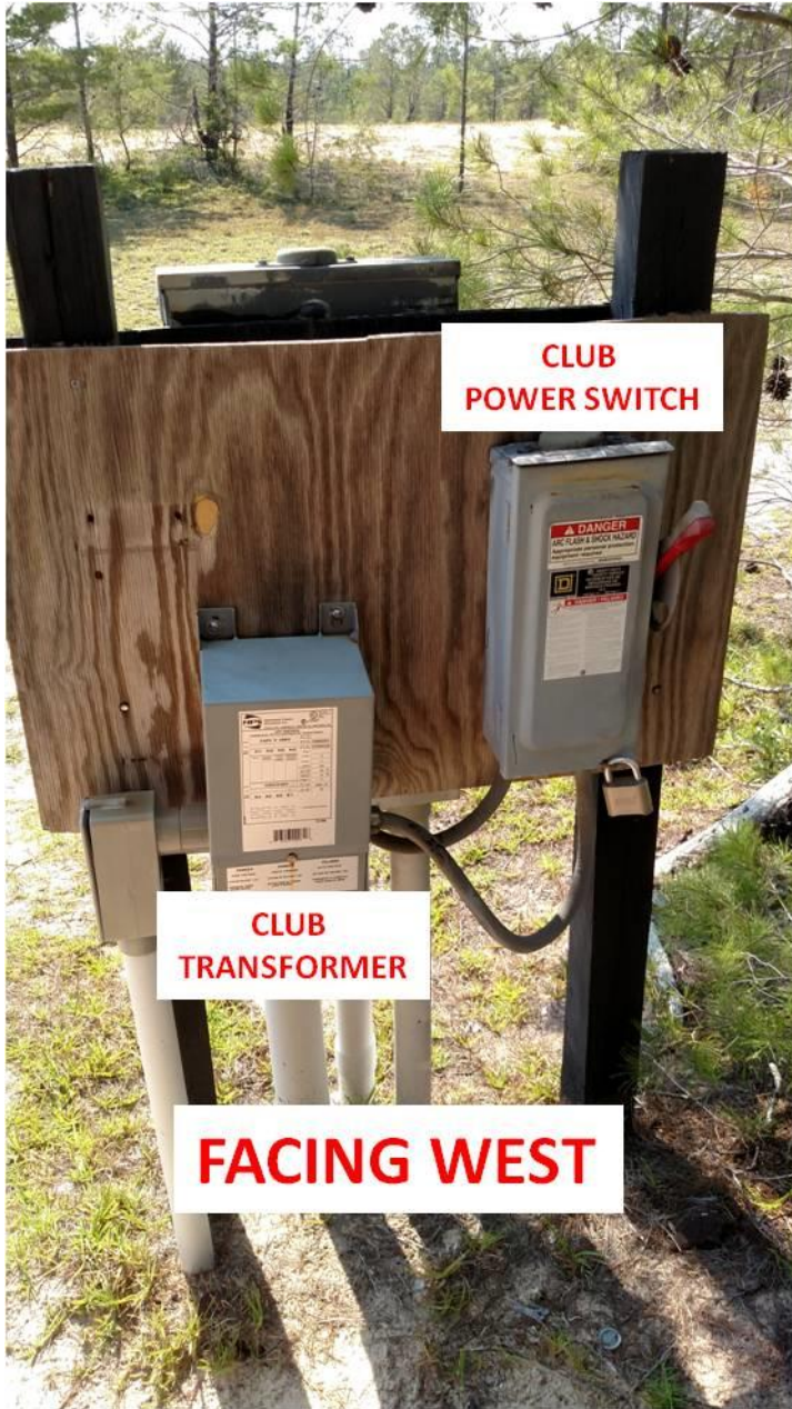
Figure 3 Club side of the electrical junction. Turn field power on and off here.
